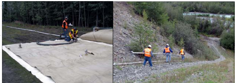
(Picture on Left) Response team preparing water bladder near location of Remote Gate Valve 108; (Picture on Right) Response team members laying out piping that would be used to pump water from the river uphill to the water bladder reservoir. Photos courtesy of John Engles/ADEC.
